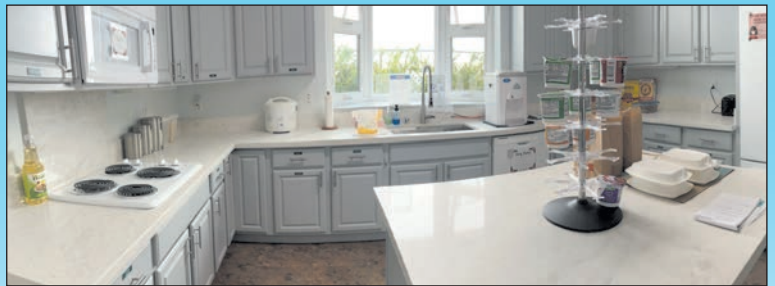
To enhance the comfortable environment for families during their stay at the Oahu Avenue Ronald McDonald House, the kitchen was remodeled and new windows were installed throughout the home that was originally built in 1998.
